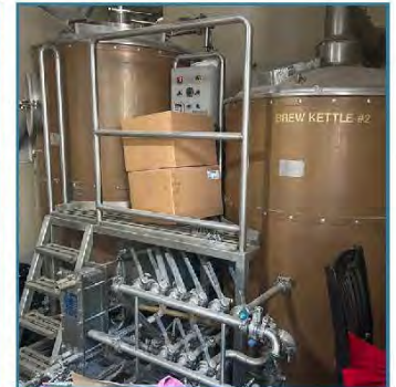
Above: Interior image of tanks
