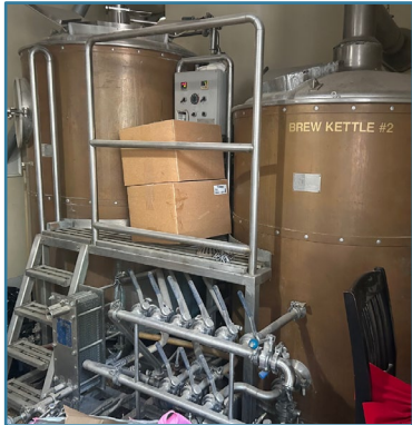
Above: Interior image of tanks
